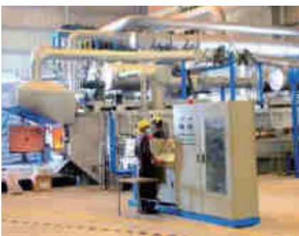
Pakistan Cables Nooriabad Factory (Pakistan)
